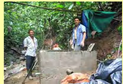
New water tanks and pipes
